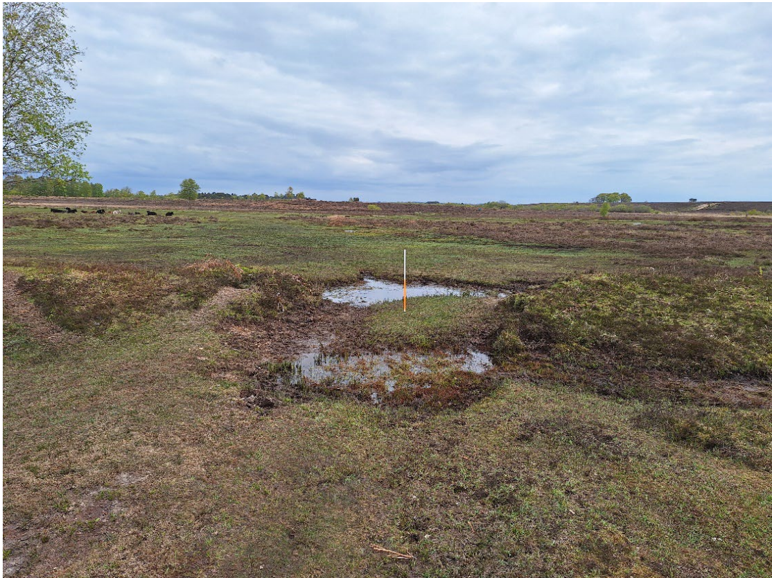
Figure 3: Breach in Bishops Dyke, facing N, April 2024 (1m Scale)
