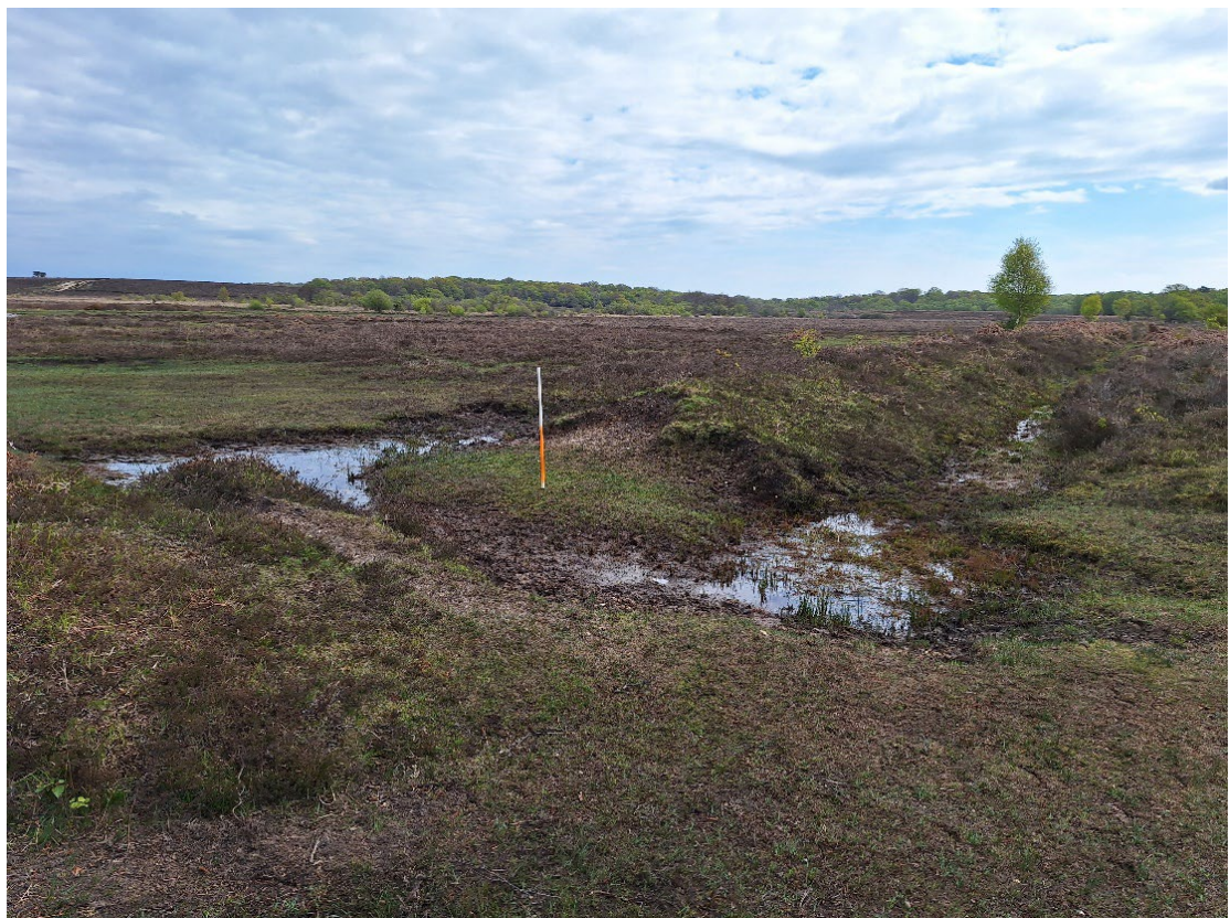
Figure 4: Breach in Bishops Dyke, facing NE, April 2024 (1m Scale)
